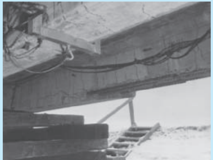
Fatigue failure of reinforcing bars in a reinforced concrete bridge.
