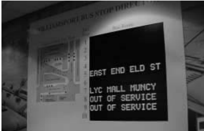
Dynamic message sign in River Valley Transit Centre, Williamsport, Pennsylvania, includes site map (left), bus bay numbers (center), and bus status information (right).
