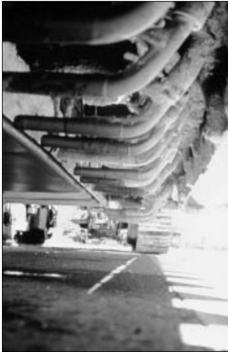
FIGURE 2 Bank of vibrators on a concrete vibration system.
