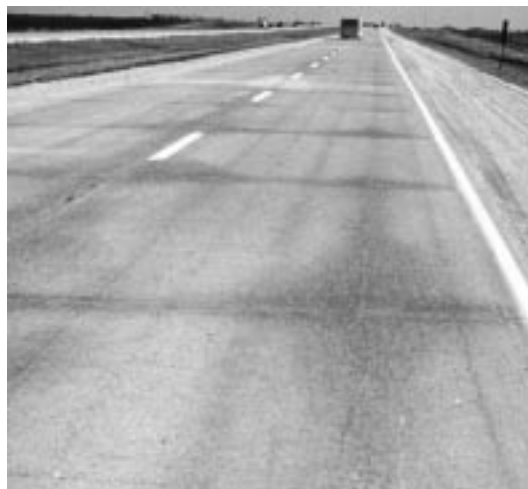
FIGURE 1 Early deterioration of concrete pavement shown by longitudinal cracks.
