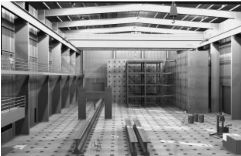
The L-shaped corner of Purdue University's civil engineering laboratory—now under construction—will feature a special floor and walls for testing large structures.
