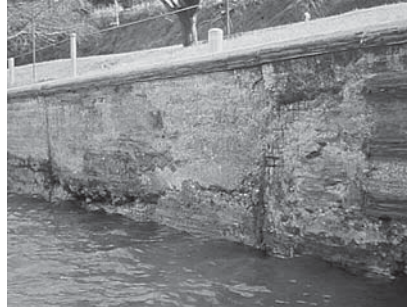
Deteriorated wall at Monongahela River Lock and Dam 3, which opened in 1907.
