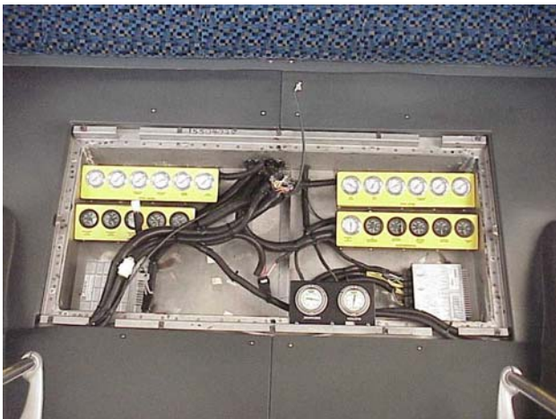
FIGURE 3 Test gauges allow for on-board systems diagnostics and training (source: DART).
