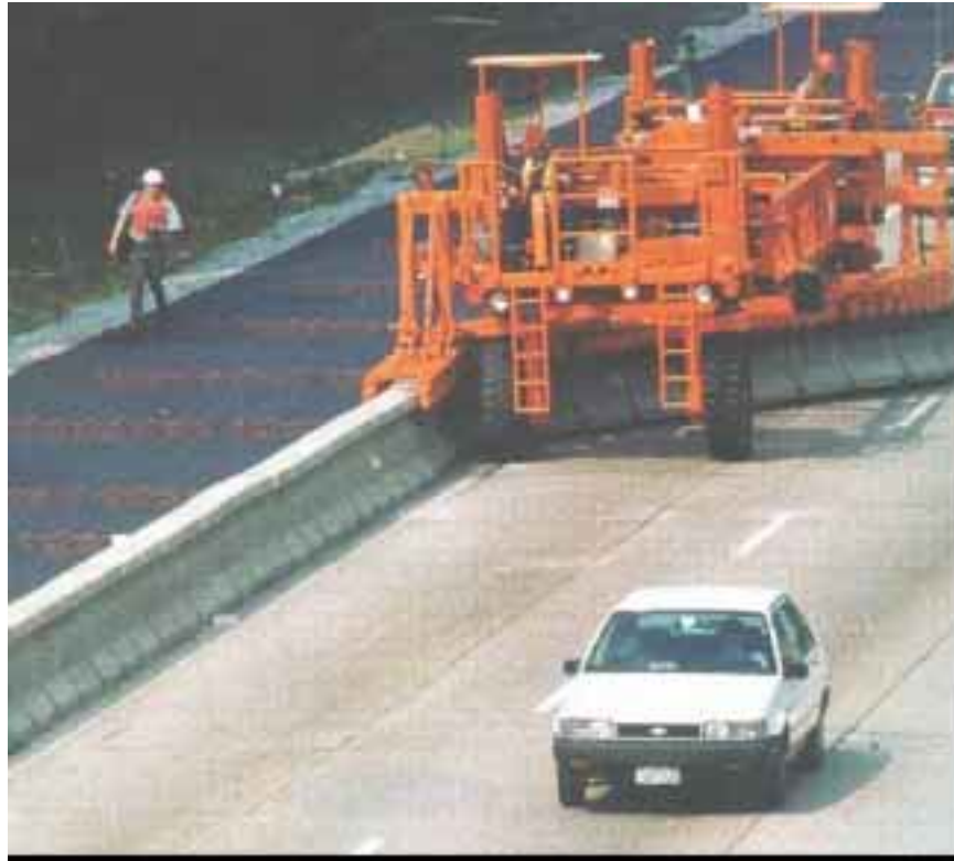
Figure B.4 Movable Concrete Barrier
