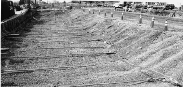
Figure 5-8. Thirty-three-year-old bars in free-draining gravel behind old quay wall unearthed at Buffalo Inner Harbor project.
