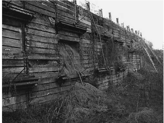
Figure 5-40. Tieback wall at TAMU-NGES.
