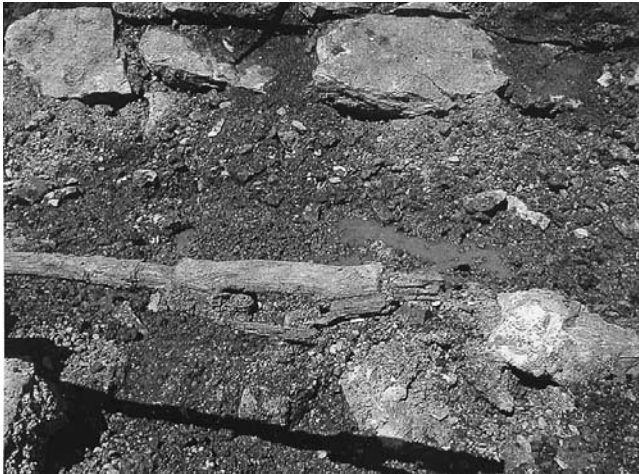
Figure 5-13. Corroded 70-year-old element backfilled in slag, exhumed at east end of Buffalo Inner Harbor project.
