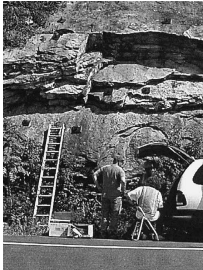
Figure 5-23. Rock slope with benches and different levels of rock bolts at Ellenville, New York.
