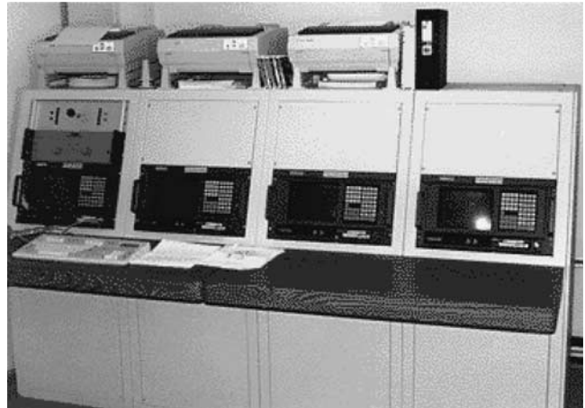
Figure 17. WesTrack control room computers.
