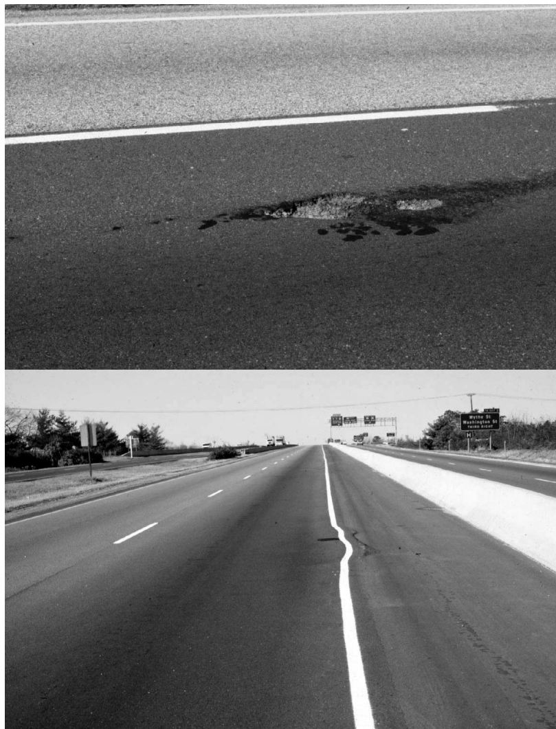
FIGURE 4 VDOT typical pavement stripping failures.
