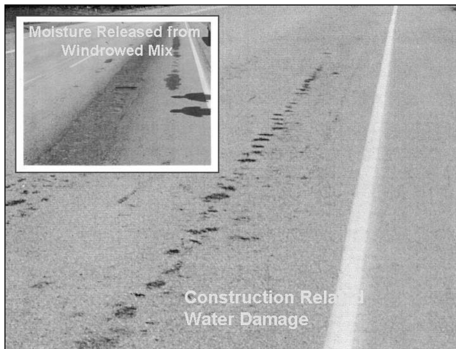
FIGURE 7 Pavement distress—localized failures.
