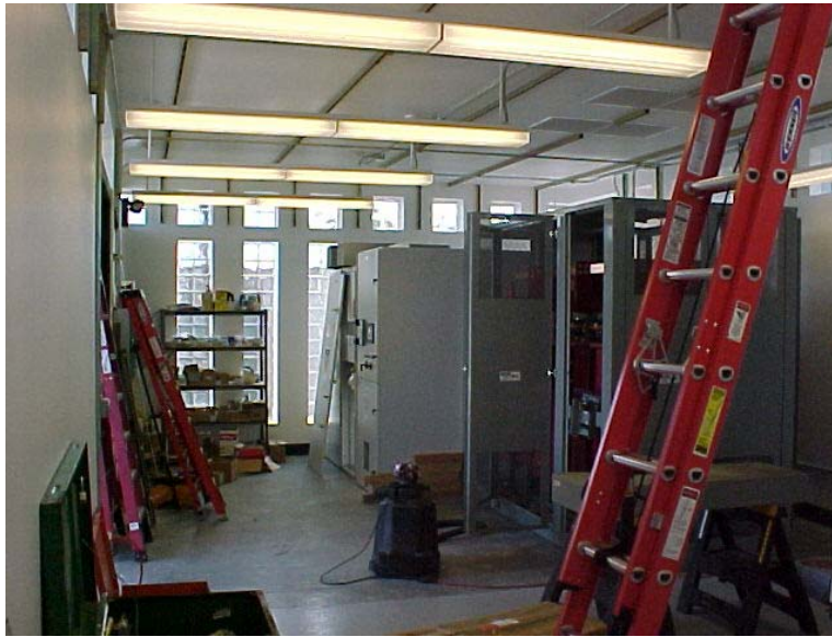
FIGURE 9 TriMet Interstate MAX LRT Expo Substation, 2003.
