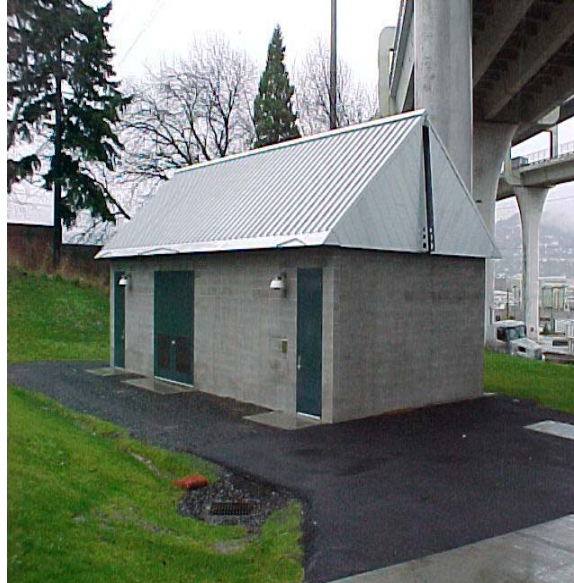
FIGURE 6 TriMet Interstate MAX LRT Graham Street Substation, 2003.
