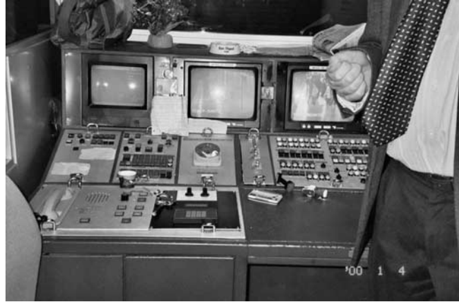
Figure 11 Station manager control booth console.
