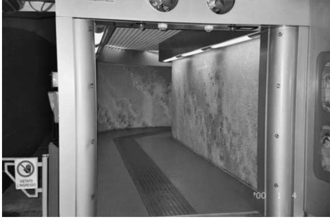
Figure 20 Station smoke/fire barrier in a station in Naples.
