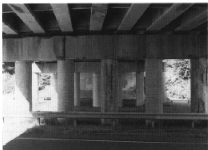
FIGURE 3-6 Concrete spalling on bridge structure.
