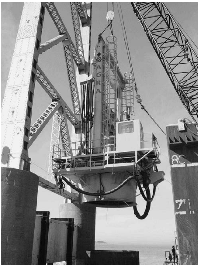
FIGURE 56 Toledo T40-4 pile top unit being placed over casing for reverse circulation drilling, Richmond–San Rafael Bridge (California) (Byles 2004).
