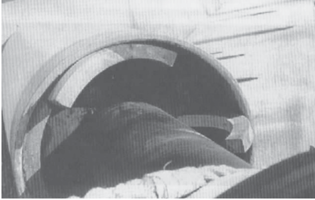
FIGURE 27 Failure of the keeper ring and dislocation of neoprene washer (Telang et al. 2000).
