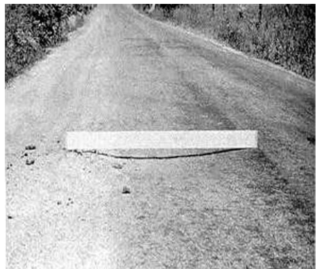
FIGURE 63 Rutting ( Asphalt Surface Treatments—Construction Techniques 1988).
