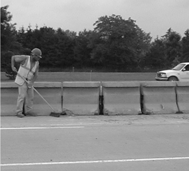
FIGURE 53 Cleaning of debris adjacent to movable barrier, Genesee County, Mich. (Courtesy: Armando Lopez, Michigan DOT).
