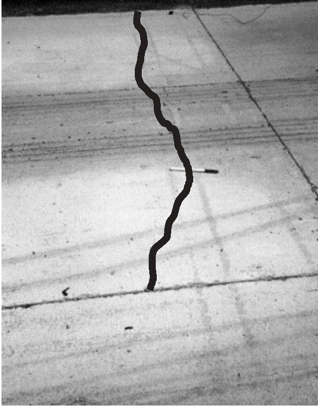
FIGURE B12 Typical UTW transverse cracking at the FHWA ALF.
