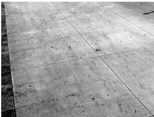
FIGURE 26 Joints without joint sealant.
