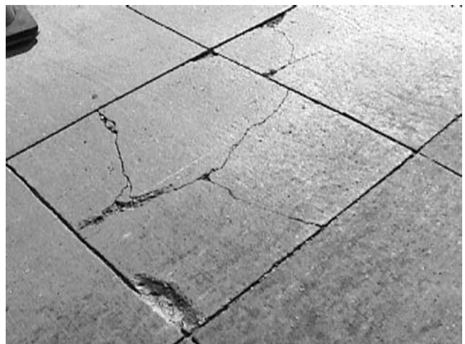
FIGURE 34 Typical shattered slab on a UTW.
