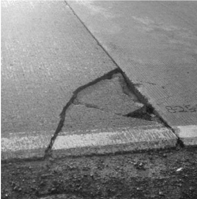
FIGURE 31 Deteriorated corner crack on a TWT.
