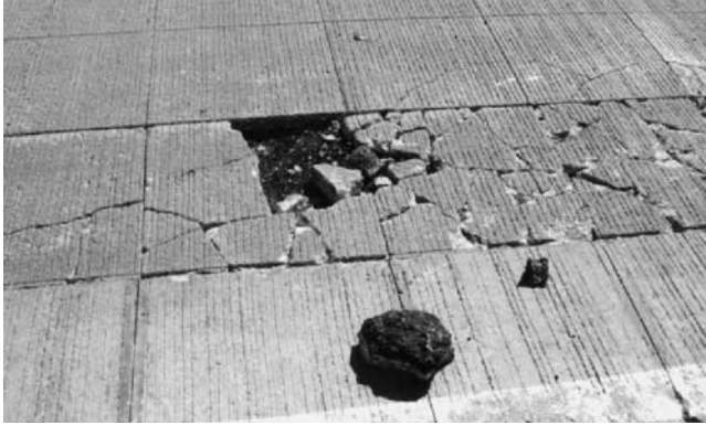
FIGURE 35 Severely shattered slabs on a UTW.
