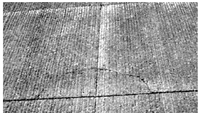
FIGURE 30 Typical corner crack on a UTW.
