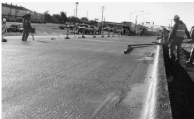
FIGURE 18 Water sheen on a concrete surface.
