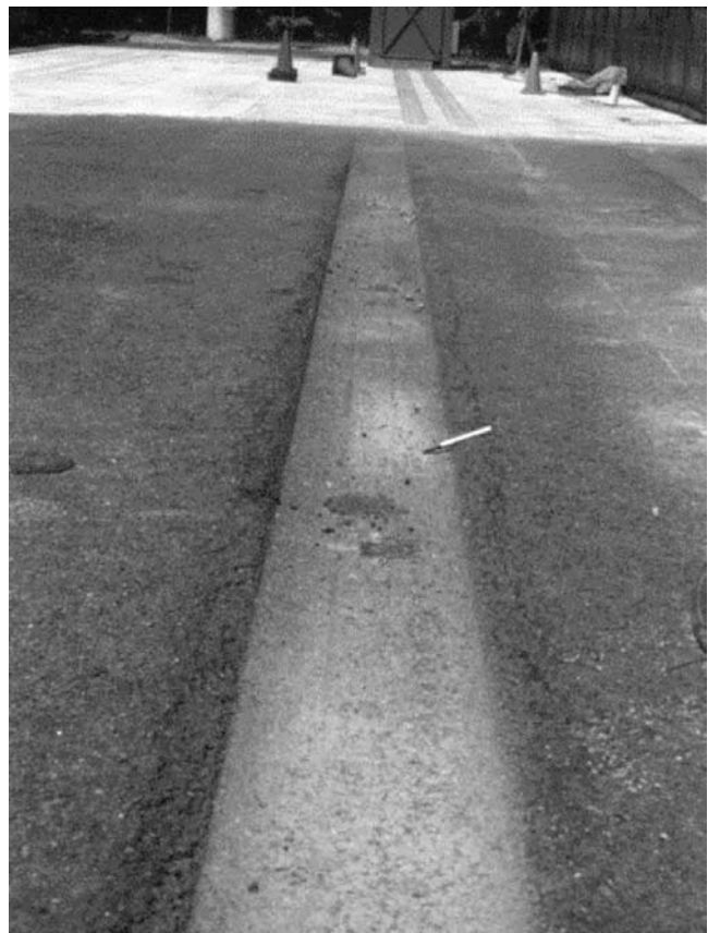
FIGURE B16 Typical HMA rutting at the FHWA ALF.
