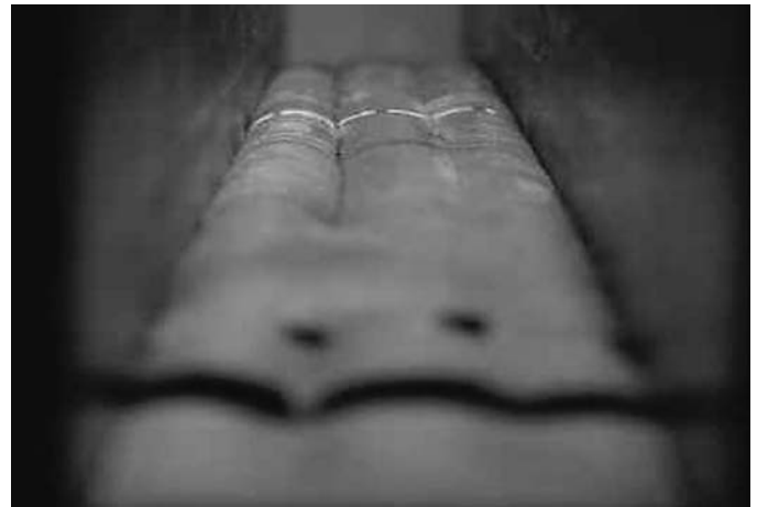
Figure 2.2. Initial debonding of bearing.
