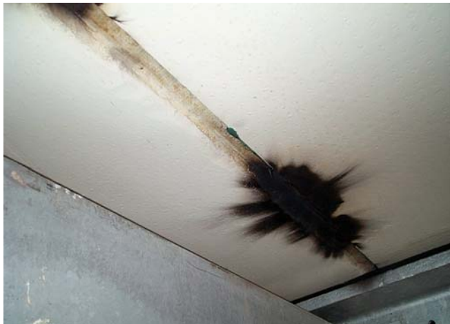
Figure 5.2.2.1-4 Attempted ignition of deck material by vandals.
