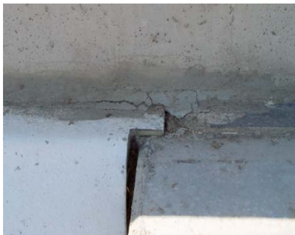
Figure 5.2.1.5-4 Concrete cracking at the parapet-to-FRP-deck interface.
