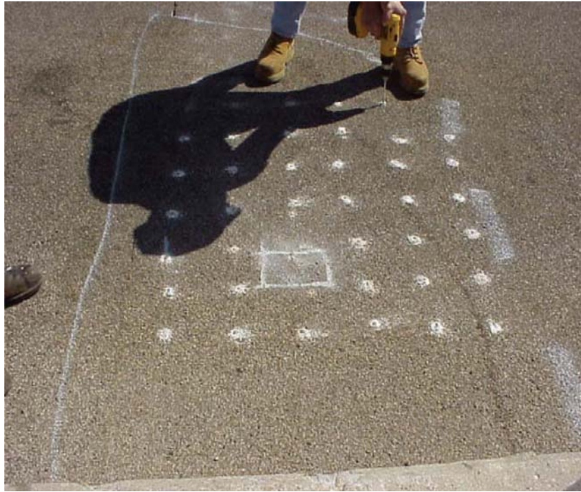
Figure 8-3 Observed blister location on deck.
