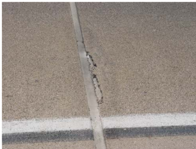
Figure 5.2.1.1-2 Debonding at joint and below wear surface.
