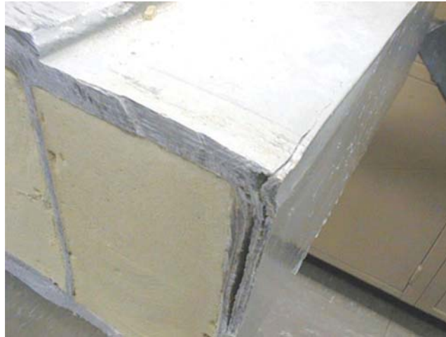
Figure 4.4.2-1 Internal voids in a closeout section of a foam-filled deck.
