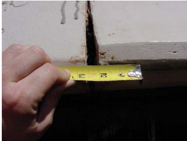
Figure 5.2.1.1-4 Misalignment of deck-to-deck joint.
