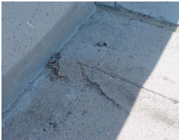
Figure 5.2.1.4-3 Buckling of wear surface on FRP deck.
