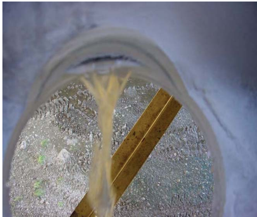
Figure 8-10 Water accumulation in cavity of deck.
