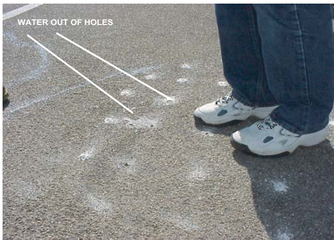
Figure 5.2.2.1-5 Water found within core of deck after drilling.
