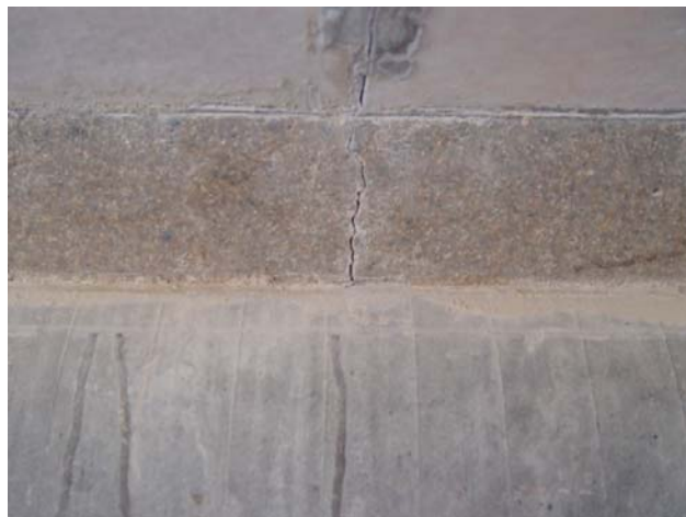
Figure 5.2.1.2-3 Crack in haunch.
