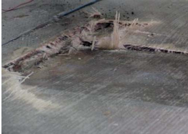
Figure 5.2.2.1-3 Punch-through of the deck from impact (Schuyler Heim Bridge).
